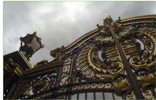
Steel Gate, Doors
